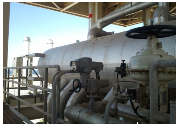
Figure (4). low-pressure heat-recovery steam generation tank in North Benghazi power station used high strength steel alloy ASTM A516-70.
