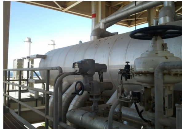
Figure (4). low-pressure heat-recovery steam generation tank in North Benghazi power station used high strength steel alloy ASTM A516-70.
